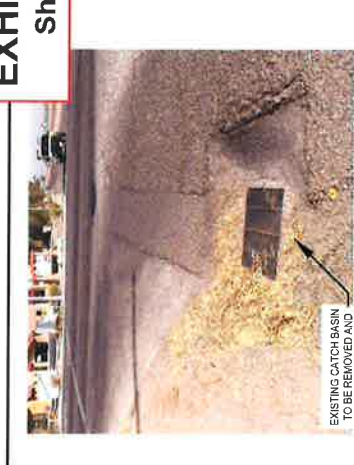
PHOTO #2 SOUTH-WEST CORNER - Labrucherie Rd & Aten Blvd Intersection EXISTING CATCH BASIN TO BE REMOVED AND REPLACED.
