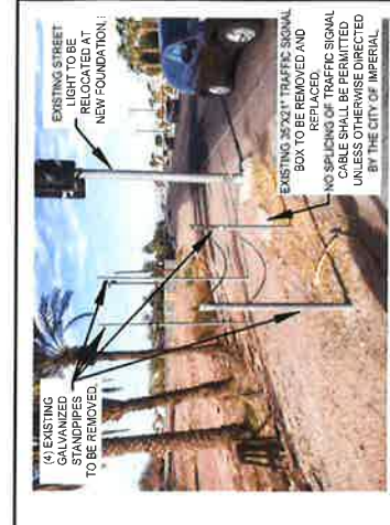
PHOTO #4 SOUTH-WEST CORNER - Labrucherie Rd & Aten Blvd Intersection EXISTING 35'X21' TRAFFIC SIGNAL BOX TO BE REMOVED AND REPLACED. NO SPLICING OF TRAFFIC SIGNAL CABLE SHALL BE PERMITTED UNLESS OTHERWISE DIRECTED BY THE CITY OF IMPERIAL.
