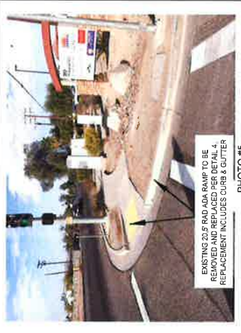
PHOTO #5 NORTH-WEST CORNER - Labrucherie Rd & Aten Blvd Intersection EXISTING 20.5' ADA RAMP TO BE REMOVED AND REPLACED PER DETAIL 4. REPLACEMENT INCLUDES CURB & GUTTER.
