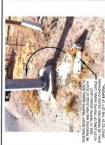
PHOTO #1 SOUTH-WEST CORNER - Labrucherie Rd & Aten Blvd Intersection EXISTING TRAFFIC SIGNAL SIGNAL BOX TO BE REMOVED AND REPLACED AT SOUTH SIDE OF TRAFFIC SIGNAL LIGHT. NO SPLICING OF TRAFFIC SIGNAL CABLE SHALL BE PERMITTED UNLESS OTHERWISE DIRECTED BY THE CITY OF IMPERIAL.
