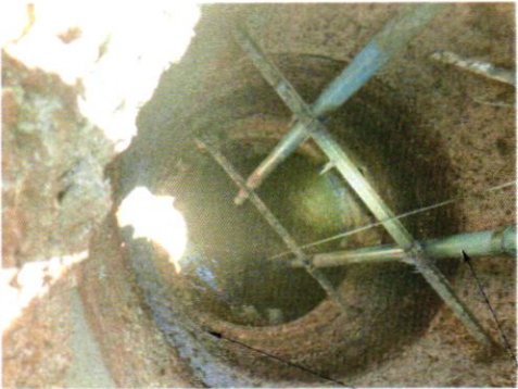
VIEW WITHIN EXISTING CROSS STREET LIFT STATION MET WELL TO BE REINBURDMENT
