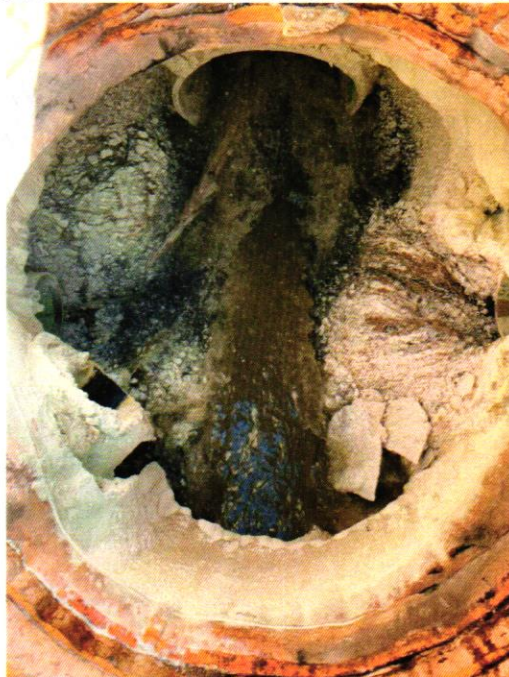
View within MH #359 to be removed and replaced with a 6' diameter manhole per Detail No. 1 on Sheet No. 3 of the bid set plans.
