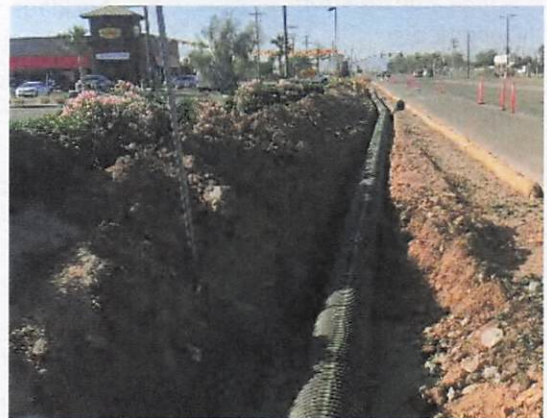
Construction of sidewalks, and necessary drainage facilities along the east side of Dogwood Avenue between Danenberg Drive and the south city limits along the out lots of the Imperial Valley Mall.
