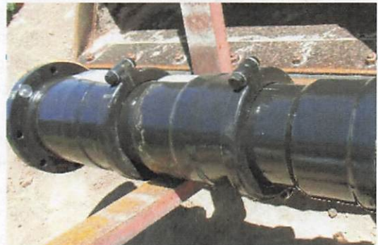
The force main project consisted of one mile of 8" ductile iron pipe connecting the Winterhaven Water District (WWD) Sewer Lift Station to the City of Yuma Sewer System and included three bridge crossings; the California Waste Way Bridge, the I-8 Over-Crossing Bridge, and the Colorado River Bridge.
