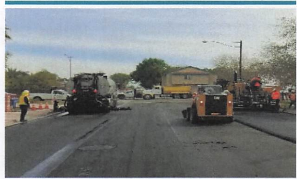
Nicklaus discovered the existing roadway section was not as described in the construction documents, leading to project quantity underruns.
