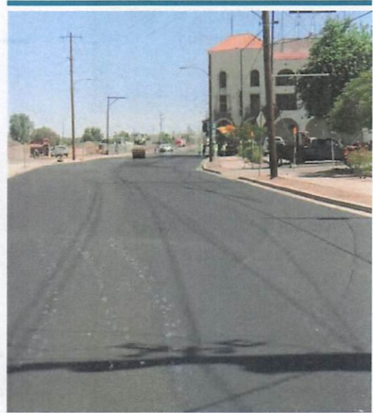
The Gila Street Improvements project consisted of improvements along four separate streets located near downtown Yuma..
