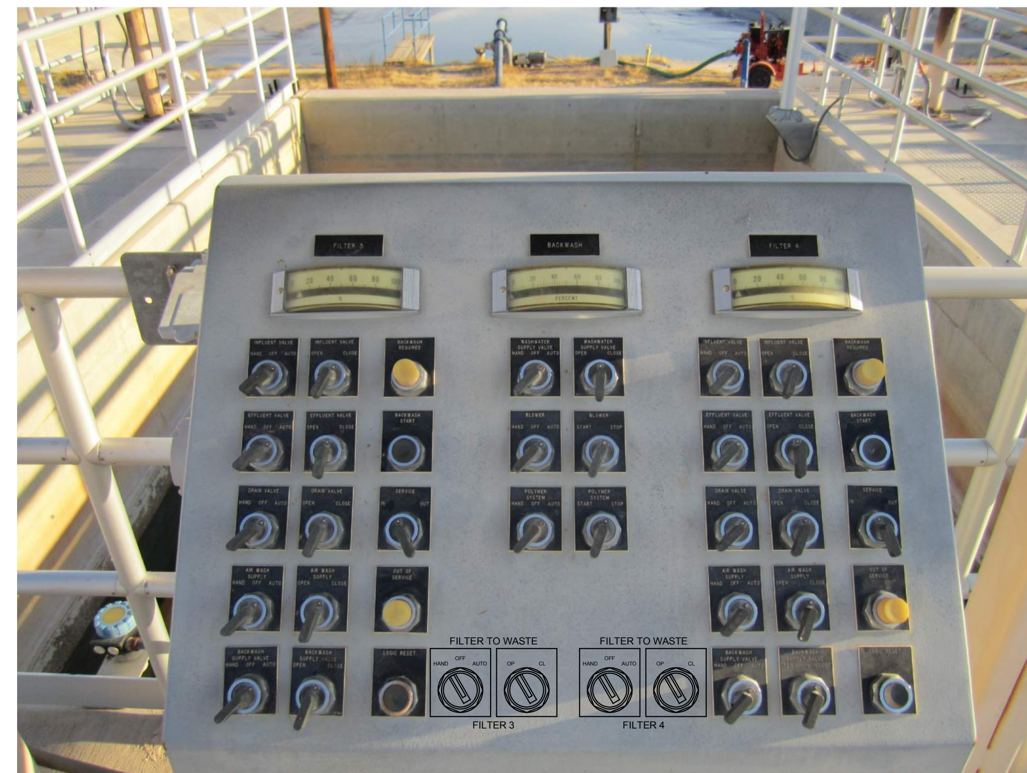
FILTER 3/FILTER 4 CONSOLE
