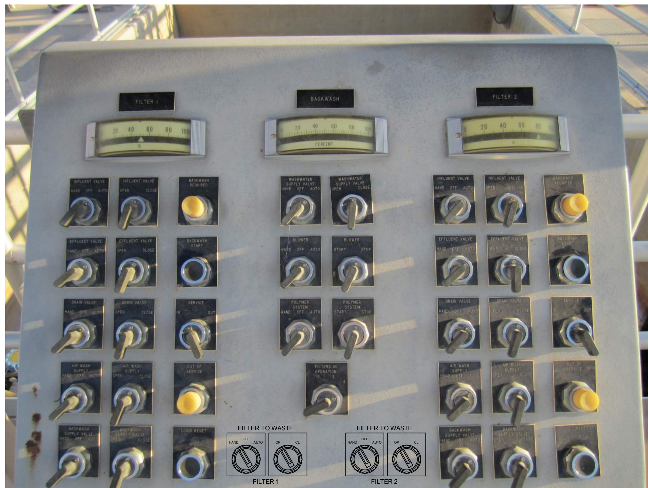
FILTER 1/FILTER 2 CONSOLE
