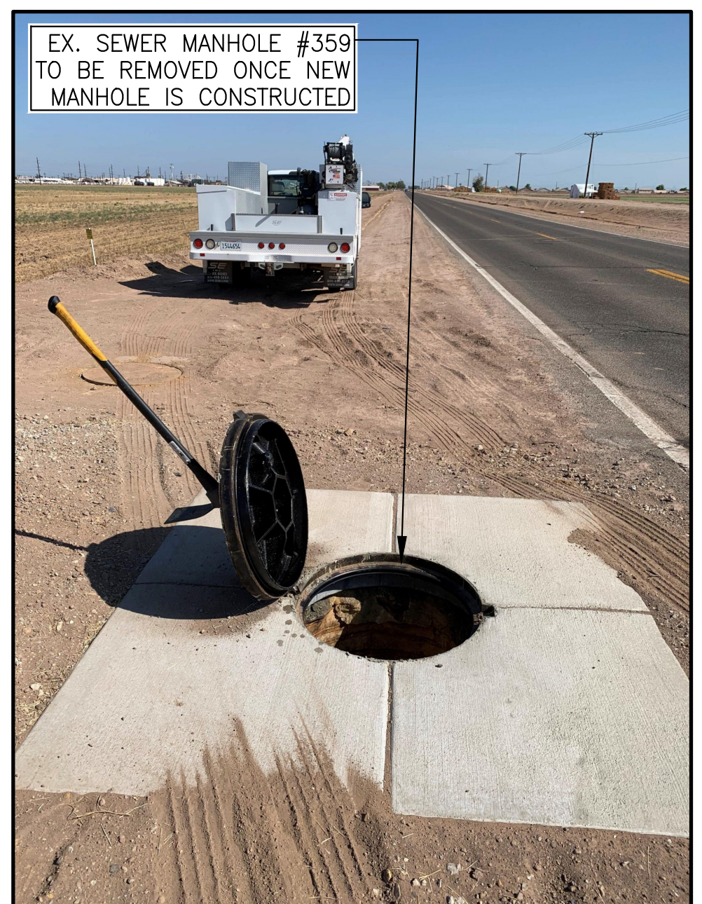
VIEW NORTH ON THE WESTERN SIDE OF CLARK ROAD TOWARD MH #359 TO BE REMOVED
