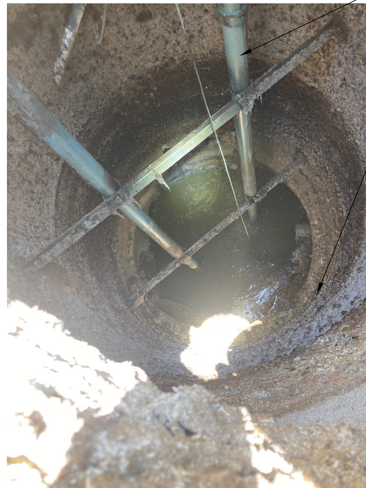
VIEW WITHIN EXISTING CROSS STREET LIFT STATION WET WELL TO BE REHABILITATED
